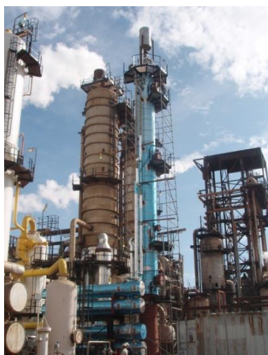
Figure 1 : Stripping unit in an oil refinery
