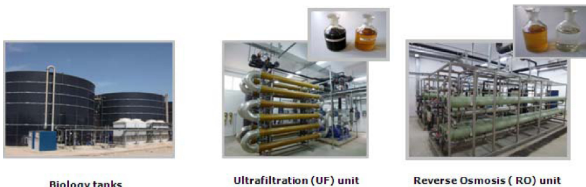
Figure 2 : DjebelChekir landfill leachate treatment plant
